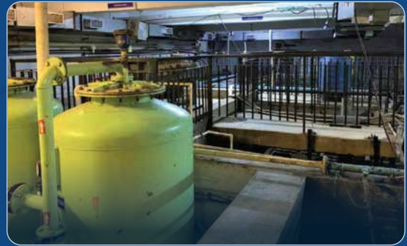
Sewage Treatment Plants (STP)
