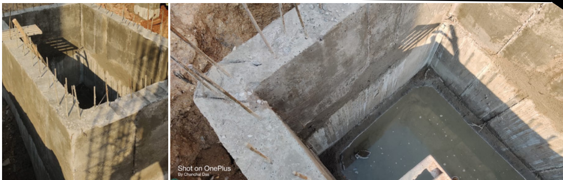
10000 LITRE CONCRETE AND STEEL ENFORCED WATER SUMP
